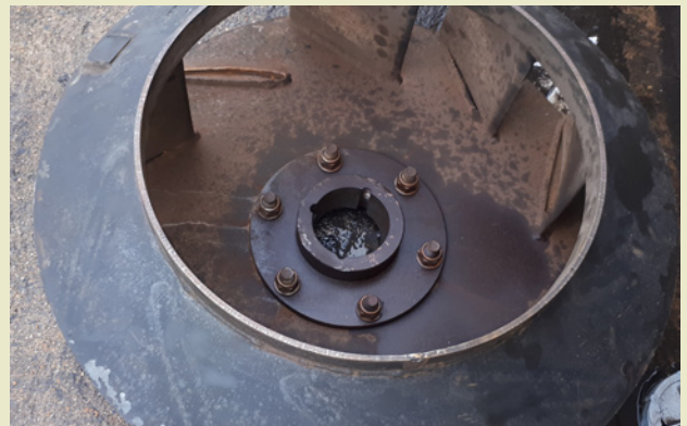
Above: The damaged combustion air fan
